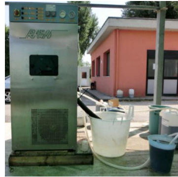
Ammonia evaporator used in two-phase hythane production process
