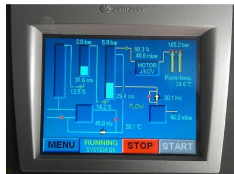
System control interface
