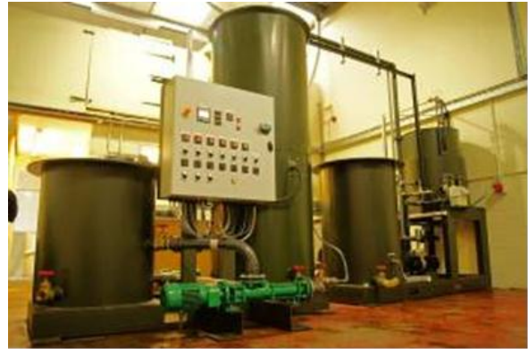
Technical scale plant used in autoclave digestion trial
