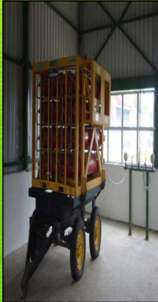
Cylinder Cascade for bottled biogas
