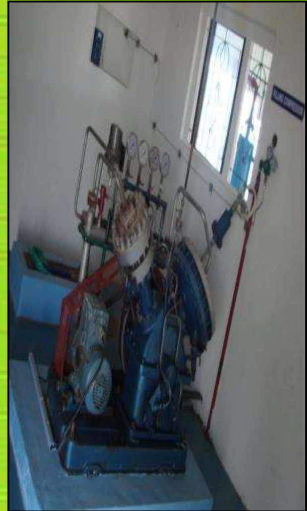
High Pressure Compressor at Nasik plant
