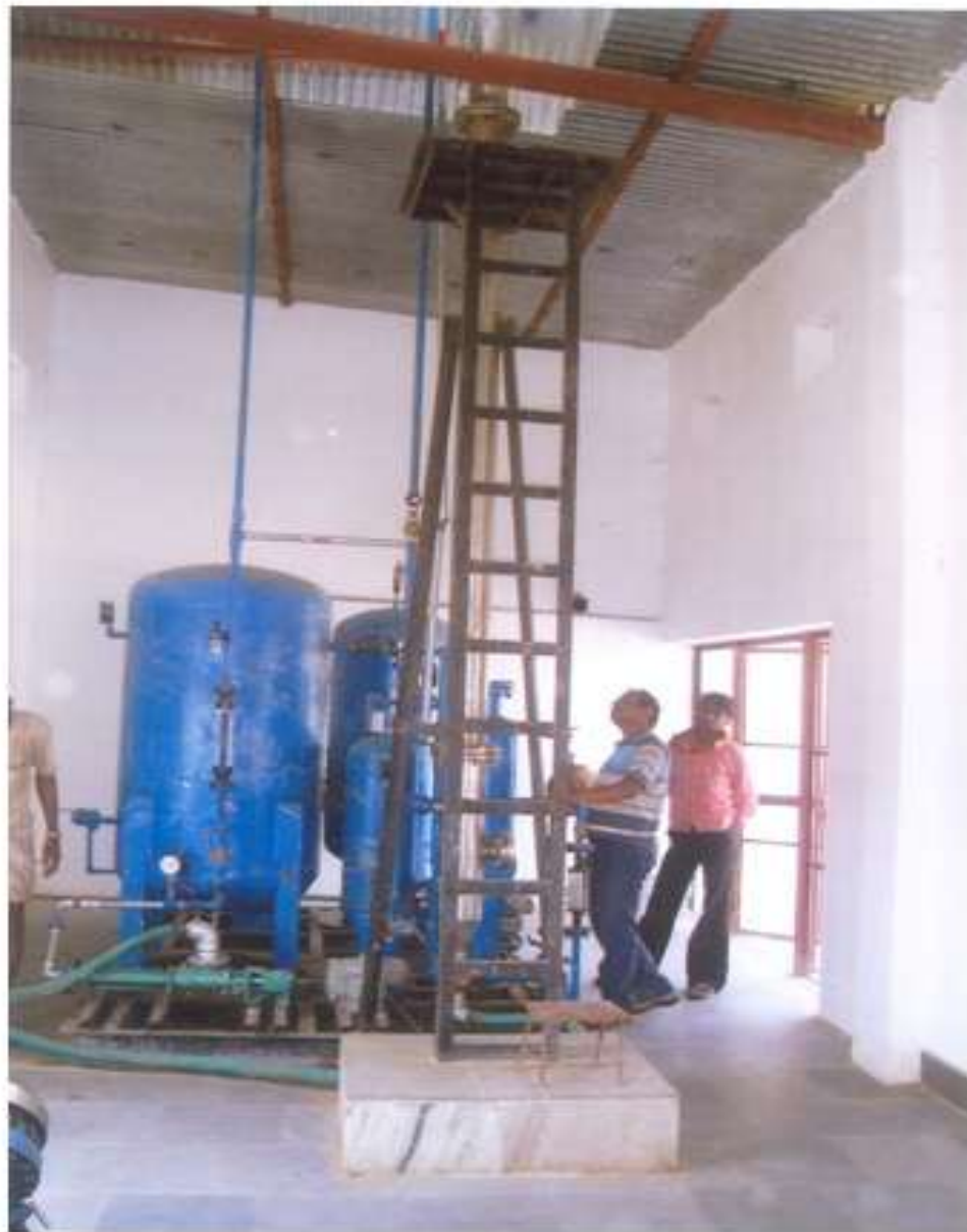
Biogas Enrichment Plant
