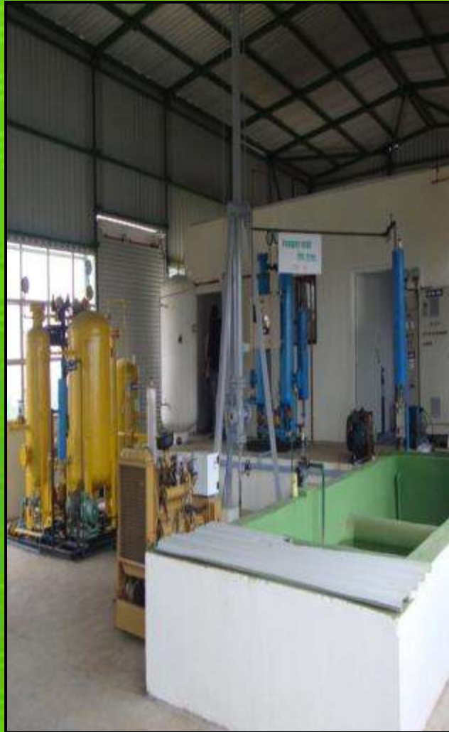
Water Scrubbing and PSA system at Nasik
