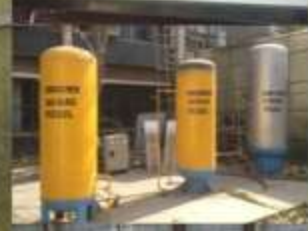
Gas Storage Vessel
