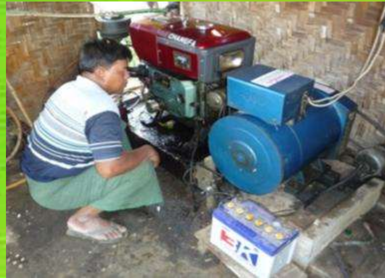
Biogas Engine for electricity production
