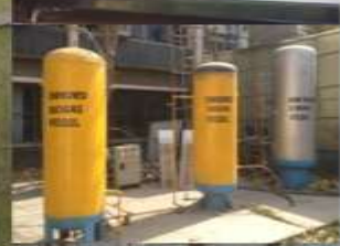
Gas Storage Vessel
