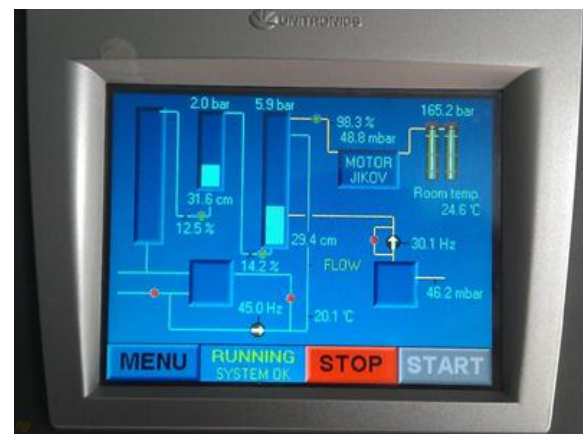
System control interface
