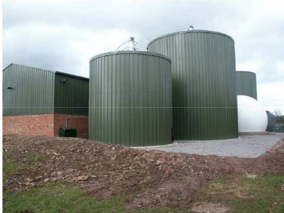
Ludlow food waste digester
